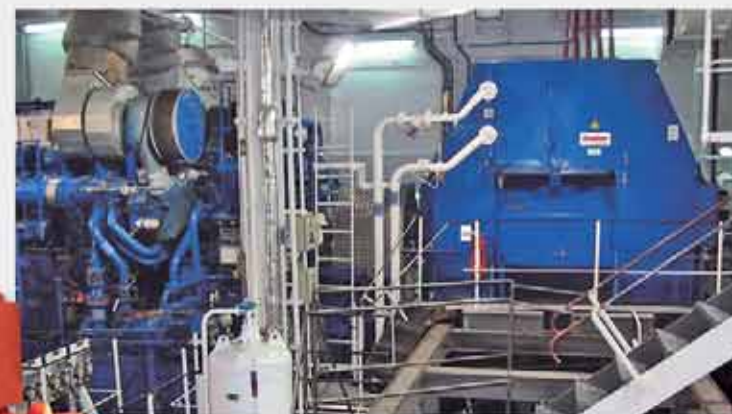
Synchronous generators, for electric needs
