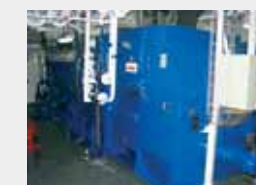
Synchronous generators, Diesel Electric propulsion
