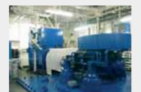
Asynchronous motors, Diesel Electric propulsion
