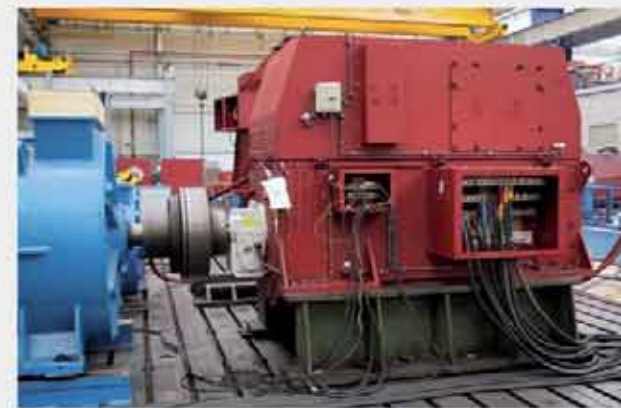
2 off main generators
